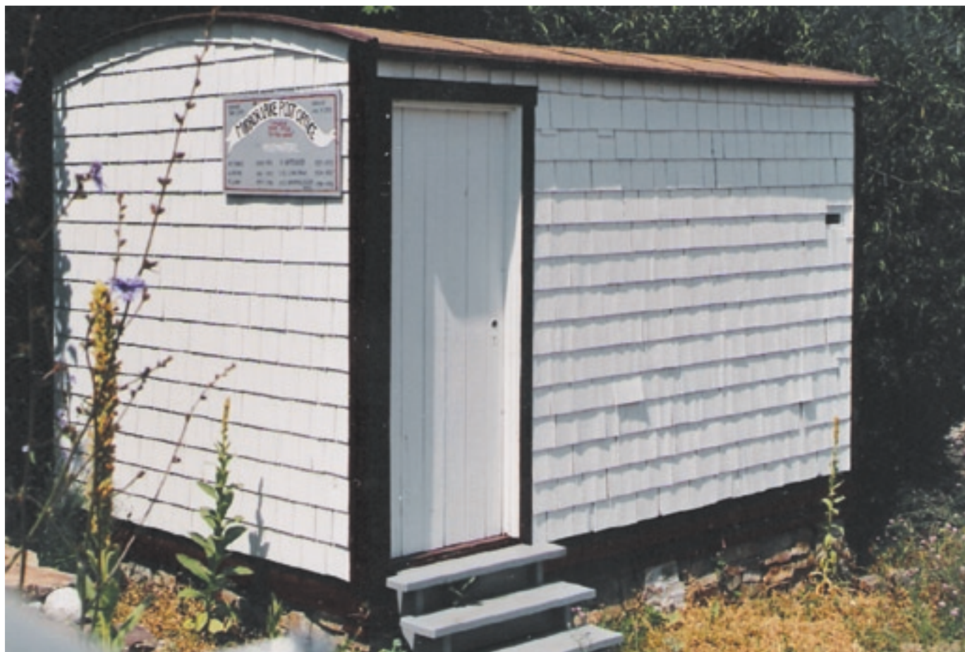
The Mirror Lake PO as it appeared in 1994. Note letter slot at extreme right of building.
